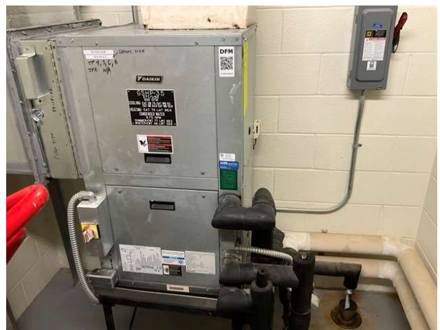
18 - WATER SOURCE HEAT PUMPS
