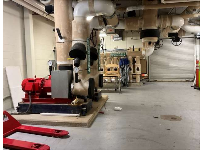
20 - MAIN MECHANICAL ROOM
