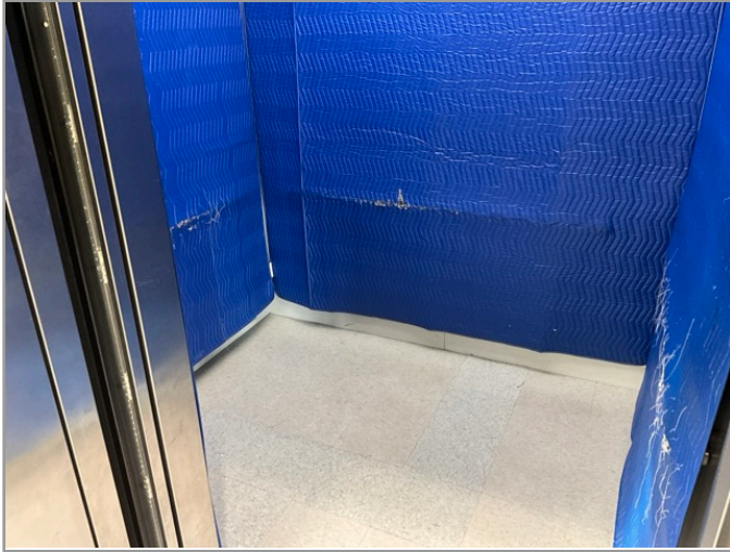
LOBBY LOOKING AT CABS (WITH DOORS OPEN)
