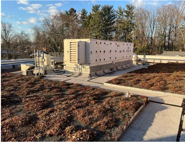
19 - ROOFTOP MECHANICAL EQUIPMENT
