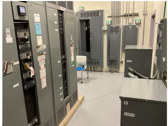
22 - MAIN ELECTRICAL ROOM
