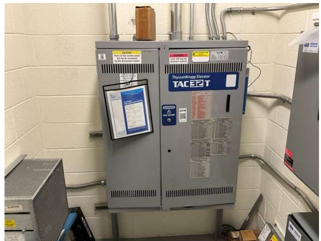
16 - ELEVATOR CONTROL ROOM
