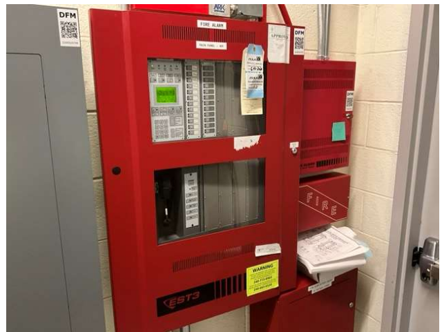
24 - FIRE ALARM PANEL
